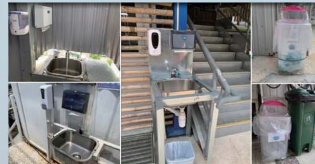
增設洗手設備及口罩棄置箱 Addition of hand washing facilities and mask disposal bins
